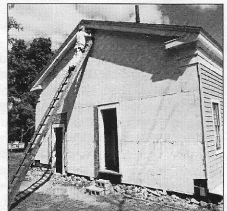
Don Randazzo restoring the back of the house after the removal of the additions.
